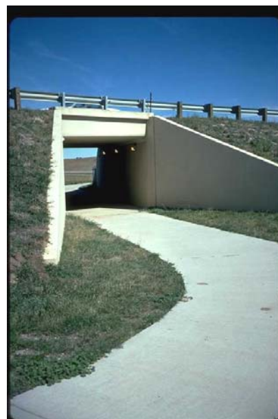
This underpass has good sightlines and approaches: cyclists can see through to the other side and the path curves gently. A mural could enhance its appeal.
